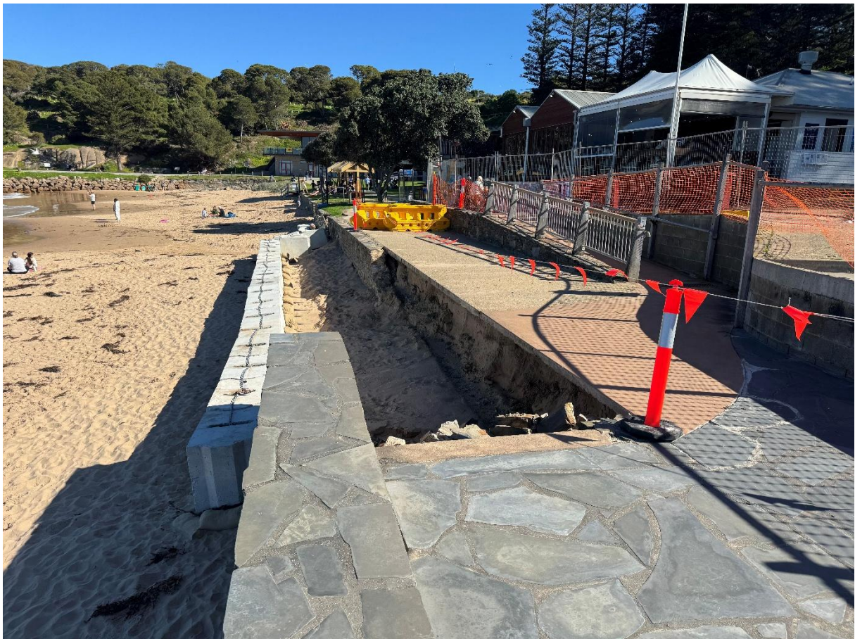
Figure 19. The destroyed seawall at Port Elliot on the 30 th August, 2026. Groundwater flow pressure blew out a section of the wall and eroded out a significant amount of sand underneath the promenade and potentially the cafe. (P. Hesp photograph).
